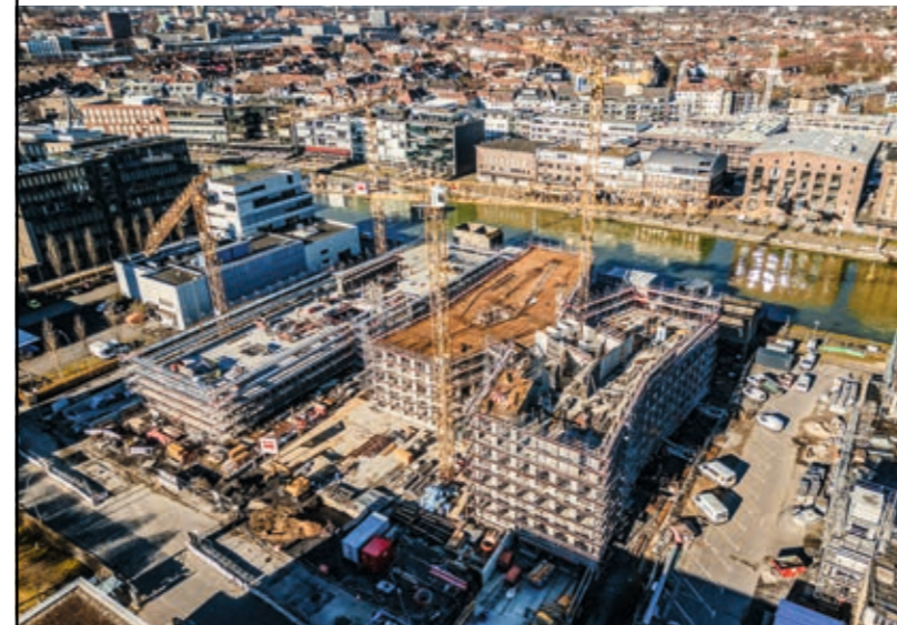
X-DOCK: Münster's Hafen district is home to the construction of an ultra-modern office building for around 500 FIEGE employees, to be completed by the summer of 2024.
